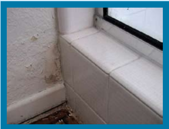
Water damage and mold growth from a leaking shower assembly.
