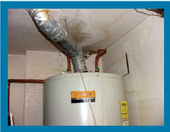
Water damage on garage ceiling from a leaking water supply line.
