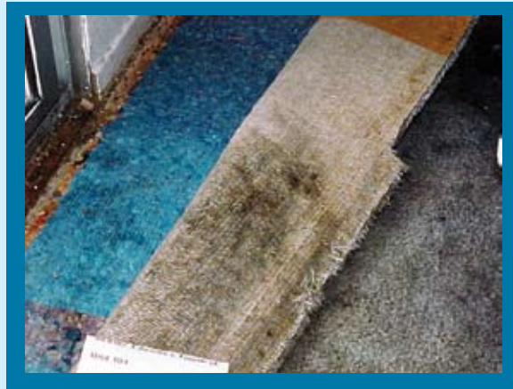
Moisture intrusion under sliding glass door causing mold growth on carpeting.
