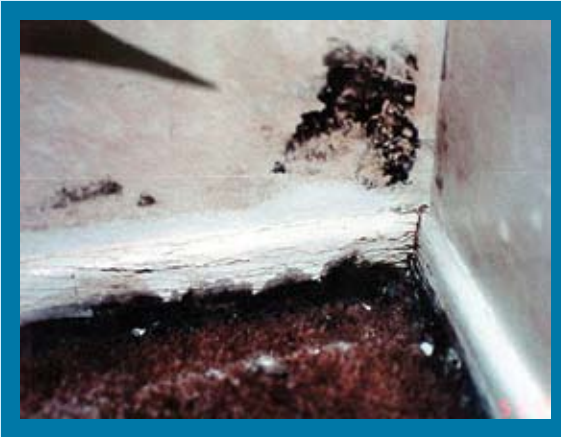
Exterior moisture intrusion causing mold growth on basedboard, wall, and carpeting.
